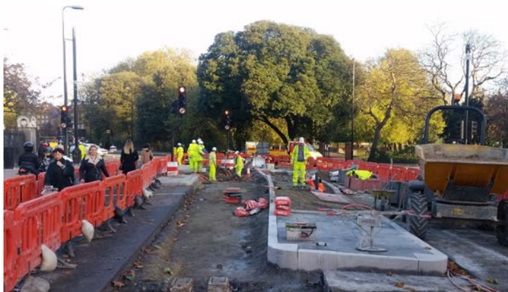
Installation of central islands on Brixton Road as part of the Oval Triangle main construction works
