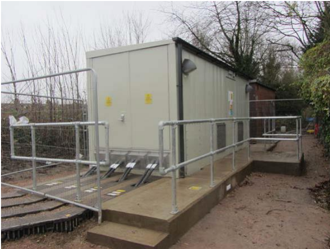
New paralleling hut at Southfields
