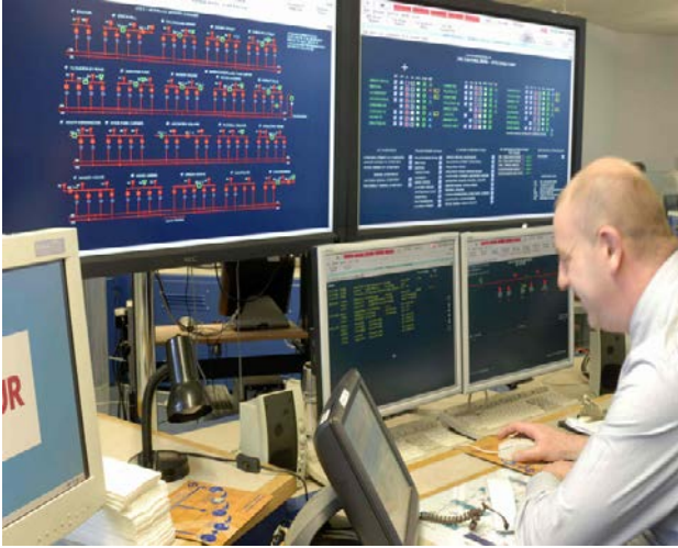
Power control room desk
